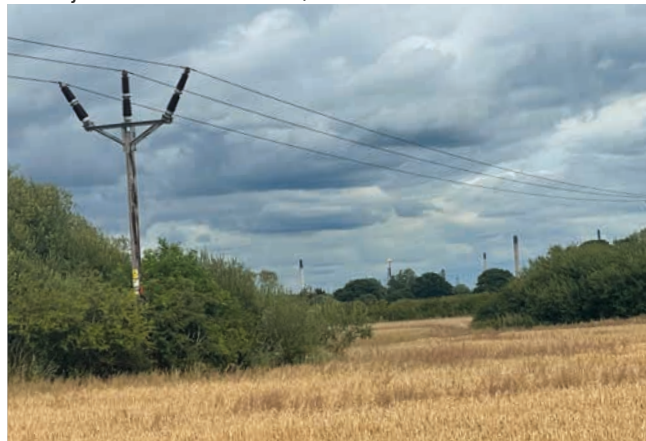
Overhead power lines
